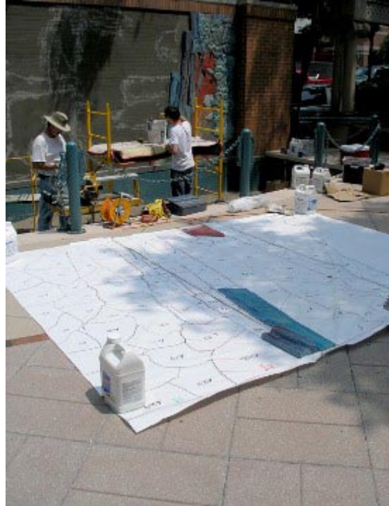
After being transported from upstate New York, the installers laid out the 500 individual, puzzle-like pieces on a numbered "map" to determine placement.
